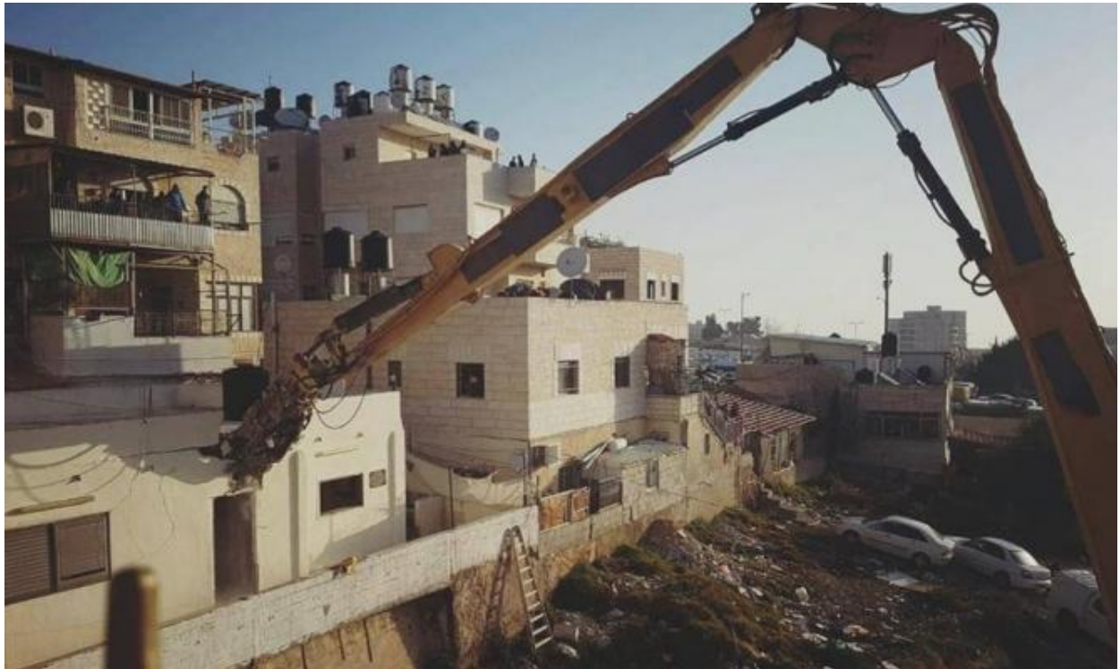
An image of a house demolition by the Israeli authorities in Beit Hanina- 2/Feb/2017
